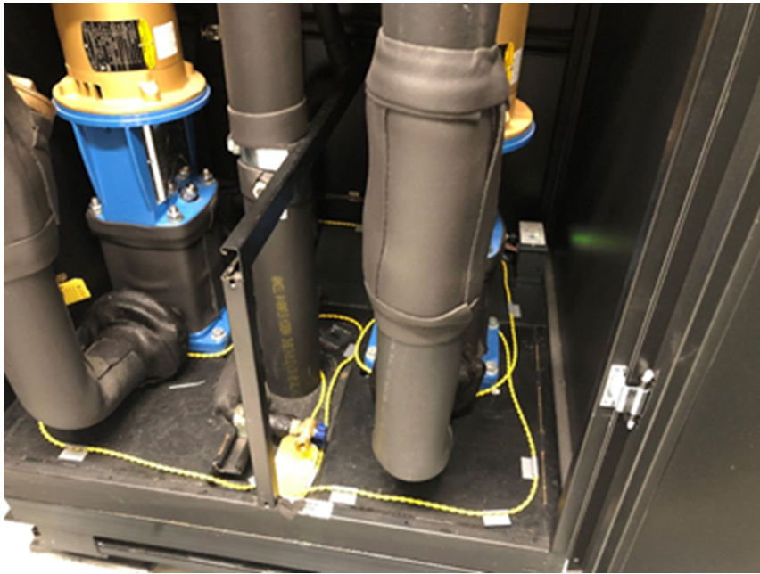
Figure 16. Leak detection rope in Vertiv® DCP 200 CDU
