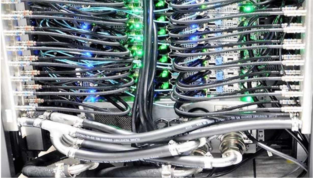
Figure 1. Rack mount CDU and dual manifold installation
