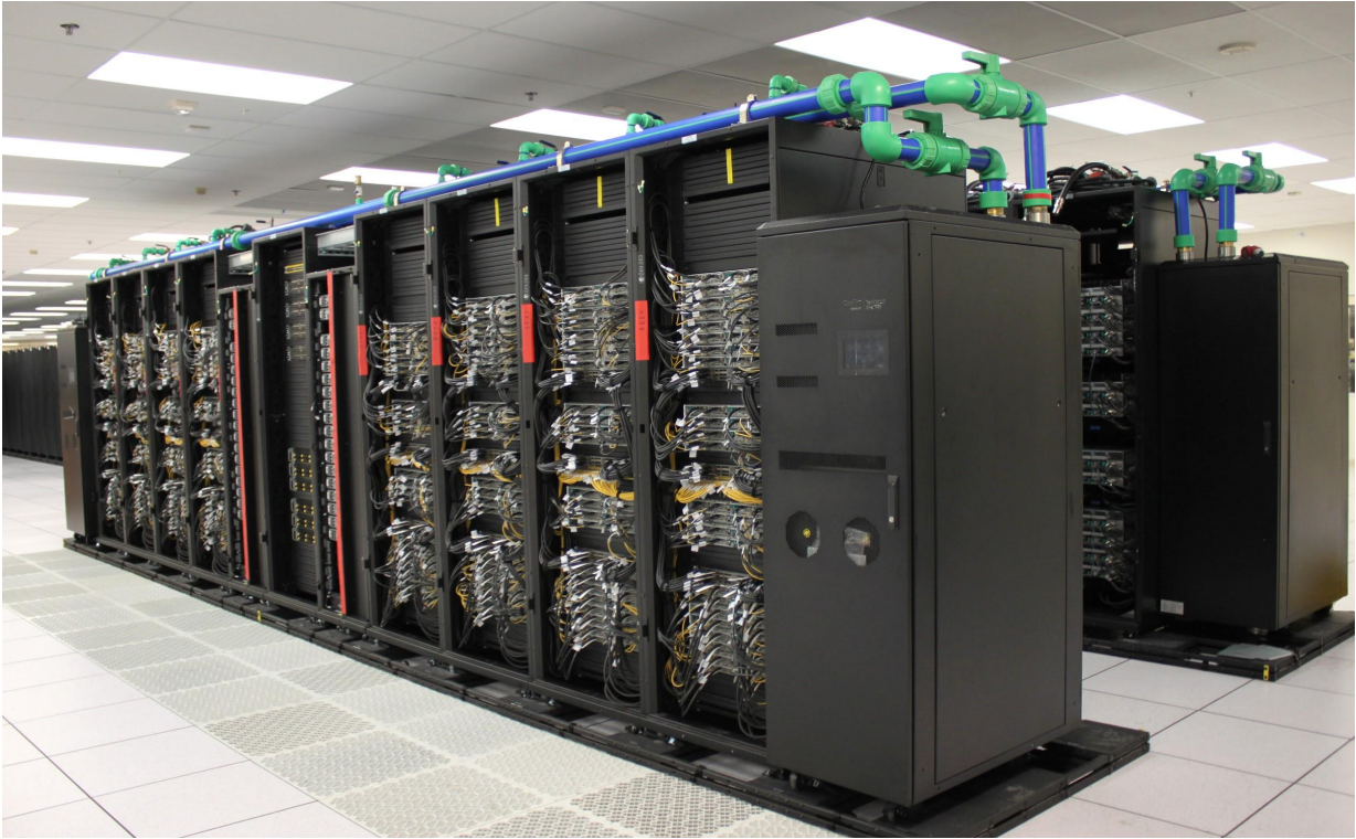
Figure 7. Above rack PP-R piping at Magma supercomputer
