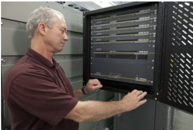
Example of a battery monitor exhibiting system data (CREDIT: ERS)
