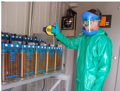
Battery Preventive Maintenance. (Credit: ERS)
