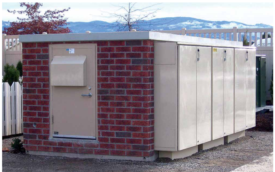
Partially Buried SmartMod CUE80 Enclosure
