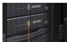
Rack sensors ensure the correct amount of cold air is provided to eliminate hot spots.
